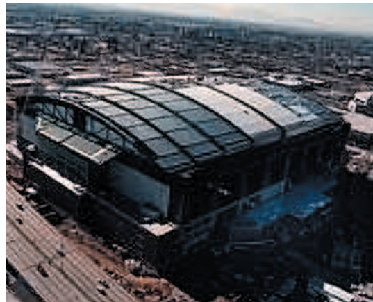
Hot Arizona weather requires state-of-the-art cooling system
