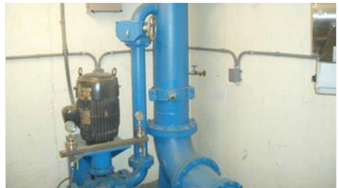
Recirculation pump and chemical injection equipment is installed in valve vault.
