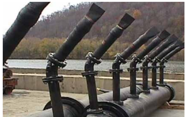
Tideflex® Effluent Diffuser Nozzles installed in inland outfall.
