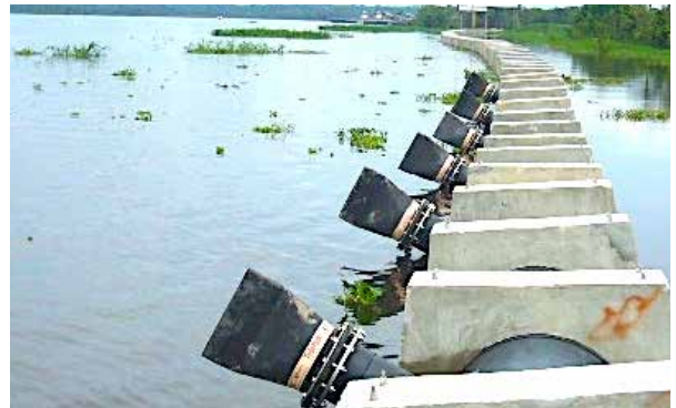
Tideflex® Effluent Diffuser Nozzles installed in marine outfall.
