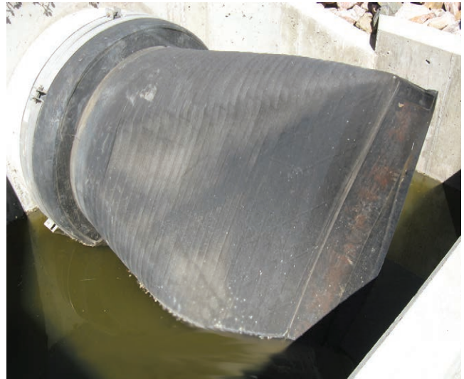
A 20" check valve with a 30" cuff, built by another check valve manufacturer. This was passed off as a 30" check valve.
