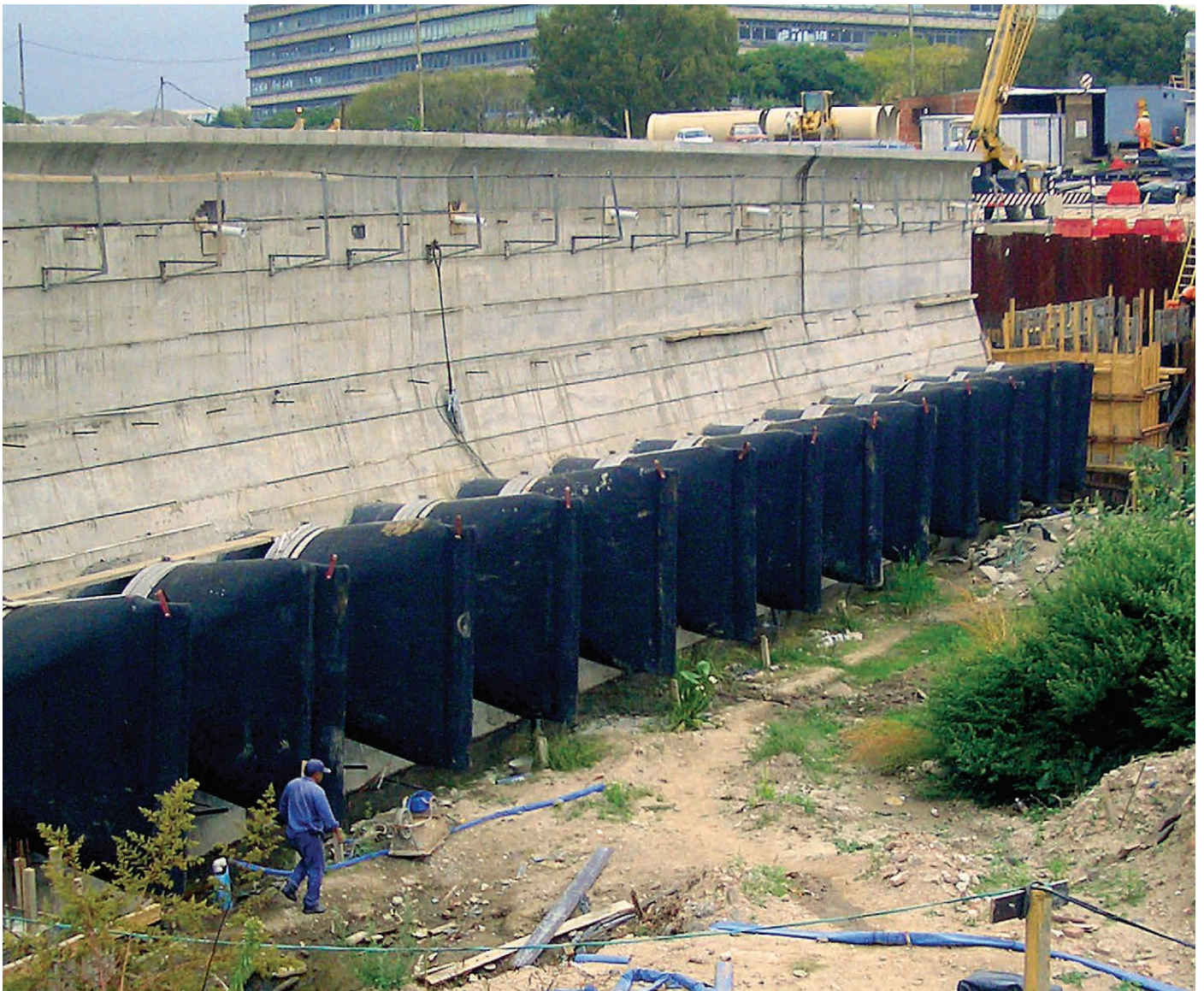
(13) 90" Tideflex® Check Valves installed in the Buenos Aires, Argentina, drainage system.
