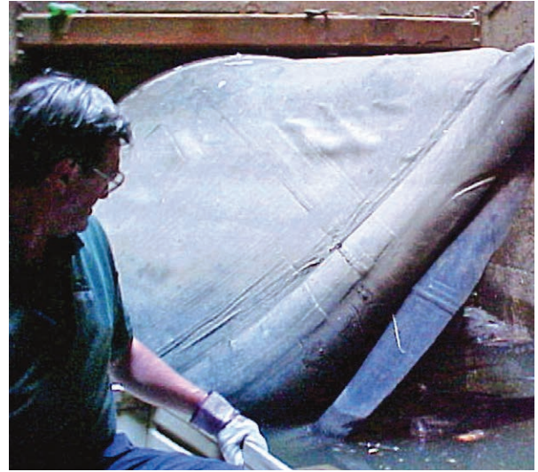
Rotating a check valve, as commonly suggested by some manufacturers, will result in distortion, gapping and leakage.
