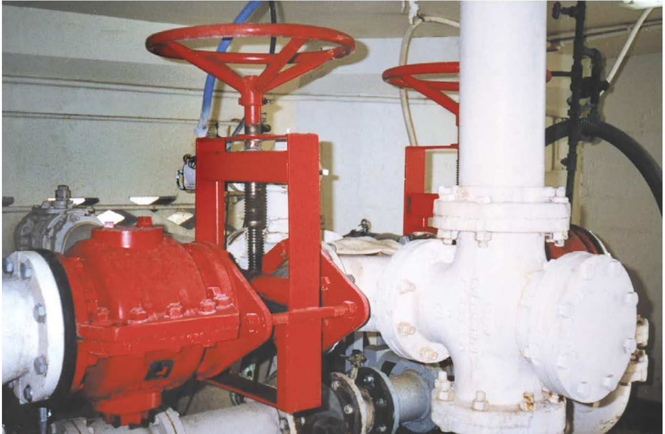
This pump station features Tideflex® CIL In-Line Check Valves (Series 39), Red Valve PVM Manual Pinch Valves (Series 70), JRE Expansion Joints for vibration absorption and SPS Pressure Sensors for accurate readings.
