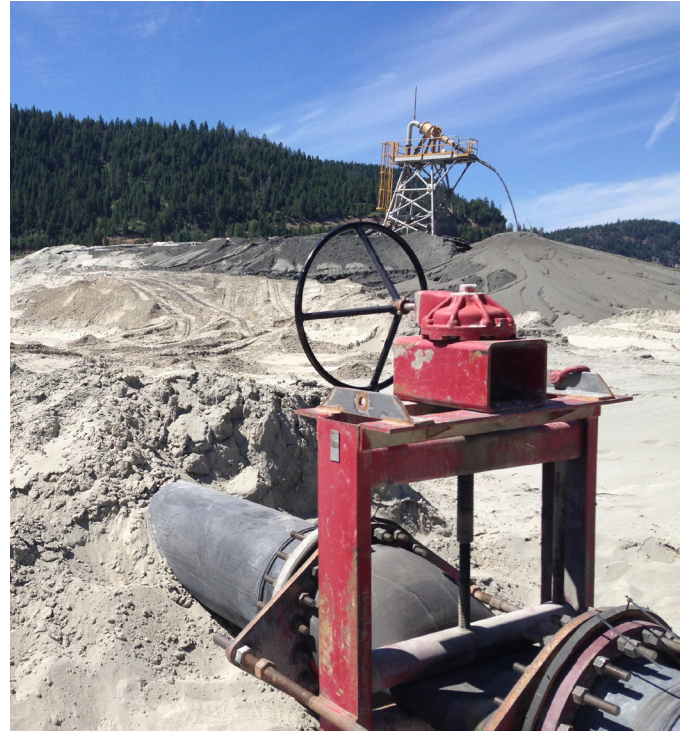
PVM - Series 70 Open Frame Manual Pinch Valve installed on a pipeline that carries rock tailings from the ore processing plant.
