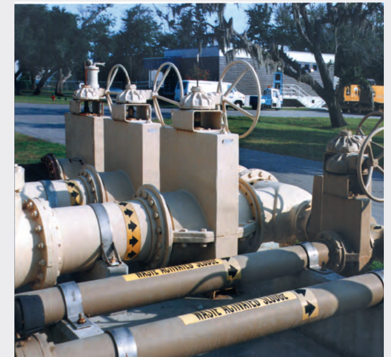
Series 75 Manual Pinch Valves installed on waste activated sludge pipelines.
