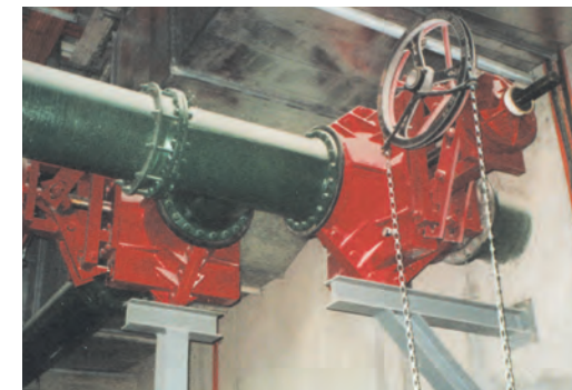
Control Pinch Valves operating at the 200 MGD Seletar Wastewater Treatment Plant in Singapore.
