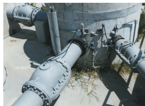
Air Actuated Type A Valves on a distribution column.
