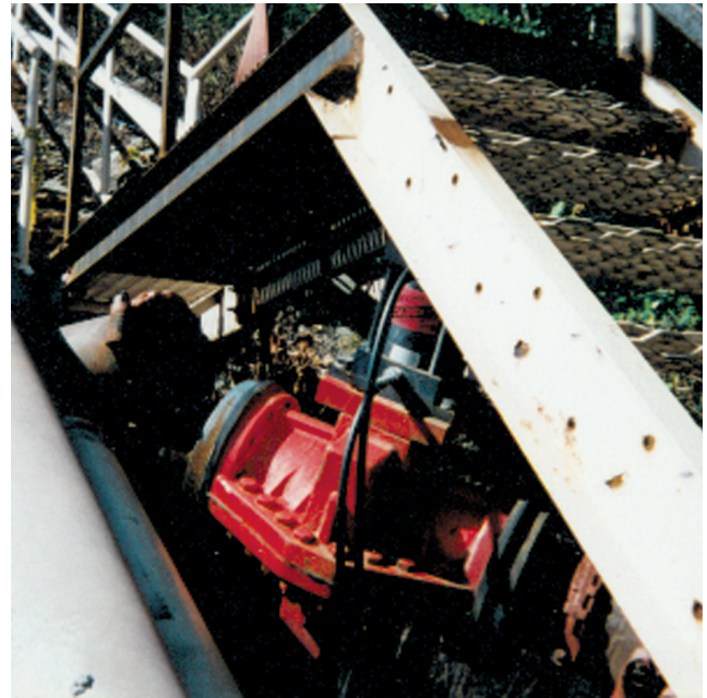
Series 9000 Hydraulic-Actuated Tailings Isolation Valve for 720 psi service at a mine in South Dakota.
