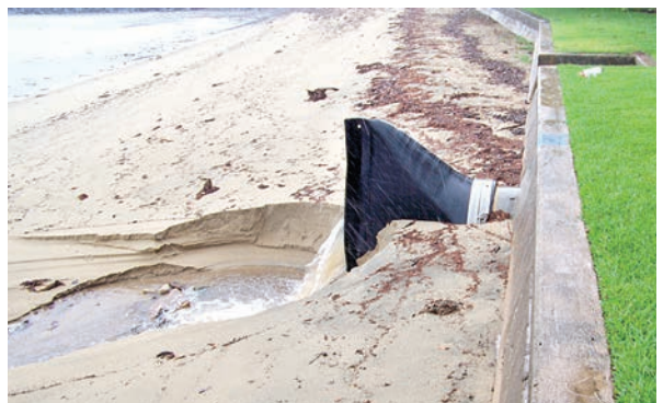
Views of Tideflex® TF-1 Check Valves installed along coastline. Note the curved bill design of the check valves does not hinder the valve's ability to open and flow in the sand.
