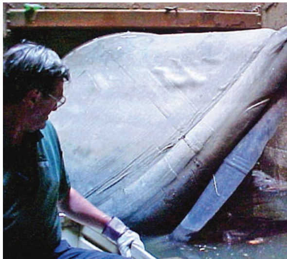
Rotating a check valve, as commonly suggested by some manufacturers, will result in distortion, gapping and leakage.
