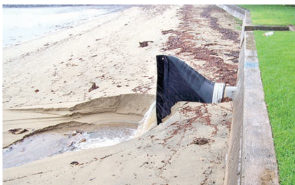
Views of Tideflex® TF-1 Check Valves installed along coastline. Note the curved bill design of the check valves does not hinder the valve's ability to open and flow in the sand.
